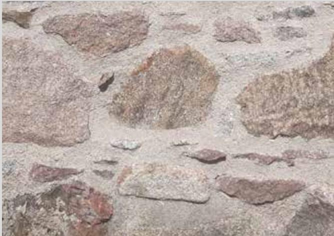
Granite rubble – Aberdeen’s oldest buildings are formed from granite rubble. These stones were hand-gathered before quarrying started. They often comprise a range of earthy colours.
