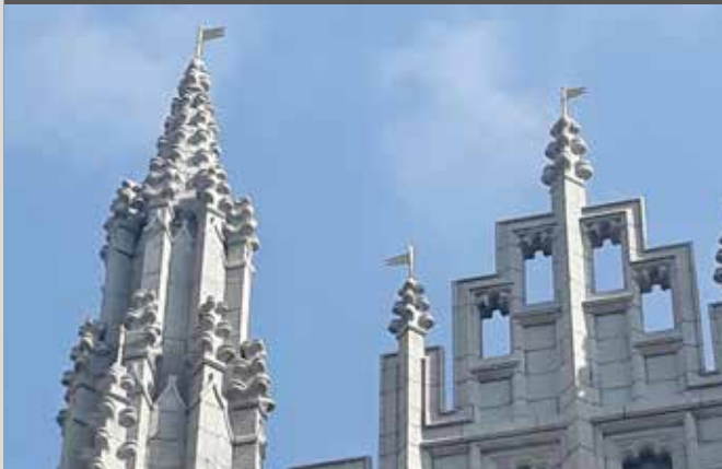
Decorative detailing – The hard-to-work nature of granite meant that decorative carvings were difficult and costly to achieve. As a result, ornate detailing is rare in Aberdeen’s buildings.
